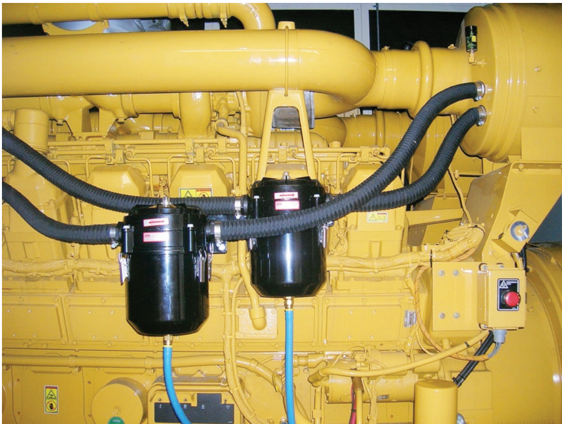
A 3516 CHD rated 2.5 mWe has a total of 3 units. 2 on one side per above. 1 on the opposite side.
